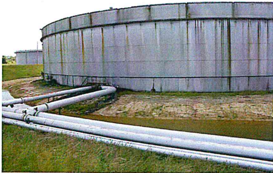
Figure B-30. Onshore Tank 102, recently refurbished, with clean bund area and aboveground pipework.
