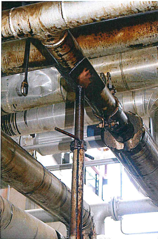
Figure B-37. Temporary pipe support in 4VDU.
