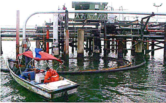
Figure B-3. Main pipe viaduct: Repair work near PB80, with Boom in the water around Sea Line 36.
