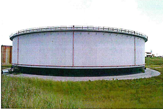
Figure B-22. Tank 103 was recently refurbished. Paint on tank and bund area look good.
