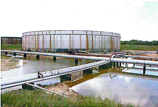
Figure B-31. Onshore Tank 101, recently refurbished, with clean bund area and aboveground pipework.
