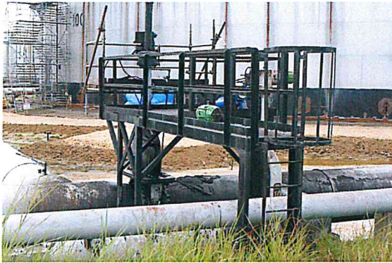
Figure B-33. Line 66 Diverter Valve at Tank 100.
