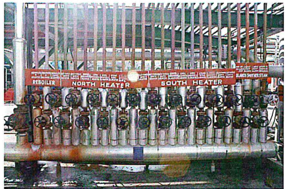
Figure B-60. Piping is labeled only at the main manifold of the unit (8CDU.)
