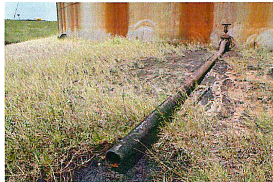
Figure B-25. Drain line piping with single valve from ground level of Tank 129.
