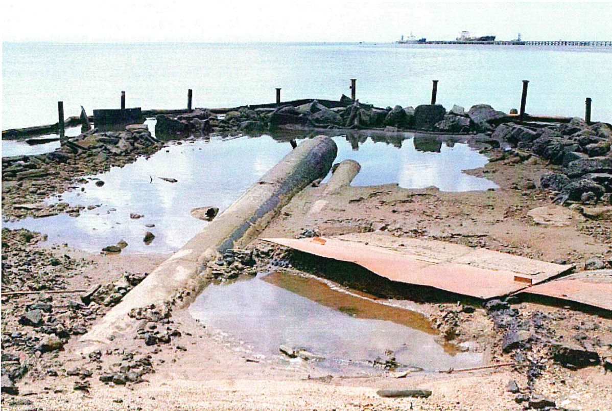
Figure B-35. Sea Line 61 at the beach between West Tank Farm and Marine Area, showing Cofferdam at area where clamp was reportedly present ca. 20 meters offshore.
