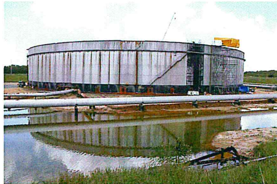
Figure B-32. Onshore Tank 100, with ongoing construction work, with clean bund area and aboveground pipework.
