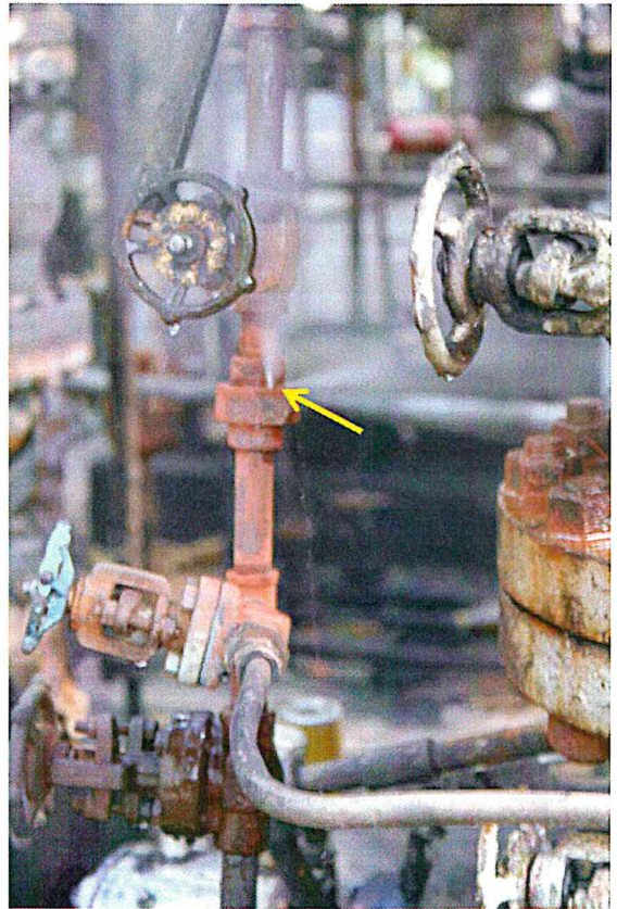
Figure B-59. Example of steam leak at threaded fitting at 8CDU.
