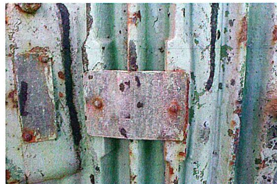
Figure B-19. Unreadable name plate on Sump Unloading Pump.
