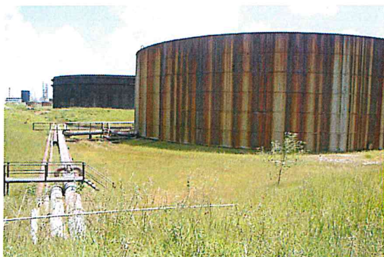
Figure B-28. Example of unlabeled transfer piping at West Tank Farm (at Tank 129.)
