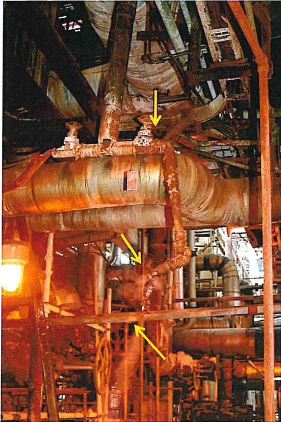
Figure B-42. Multiple steam leaks in piping of process area of 4VDU.
