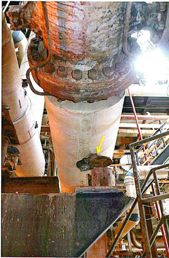
Figure B-40. Mis-aligned pipe support in 4VDU.
