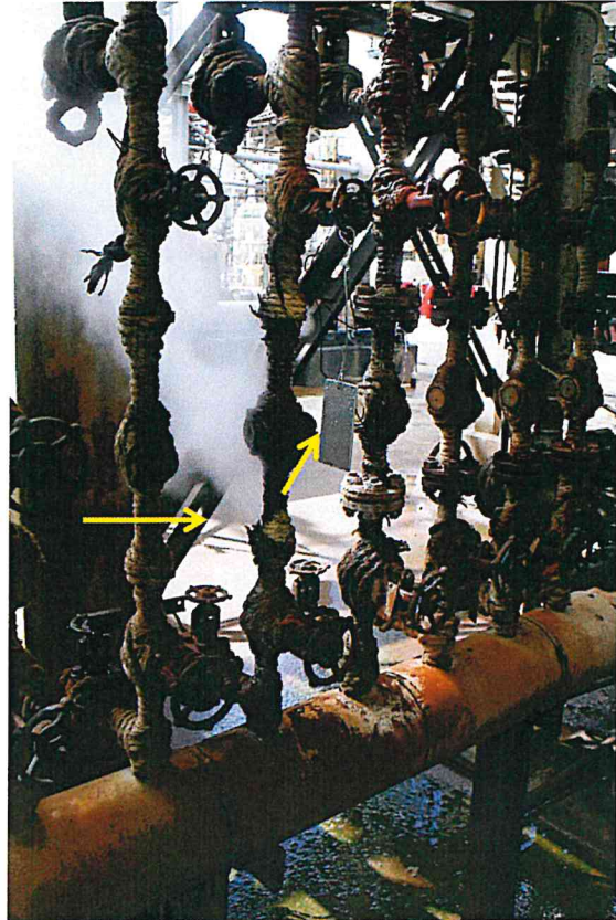
Figure B-47. Manifold with steam leak in 4VDU. Note the aluminum tag, as part of the "steam leak tagging initiative". The tag does not have any inscribed numbering to identify the leak location.
