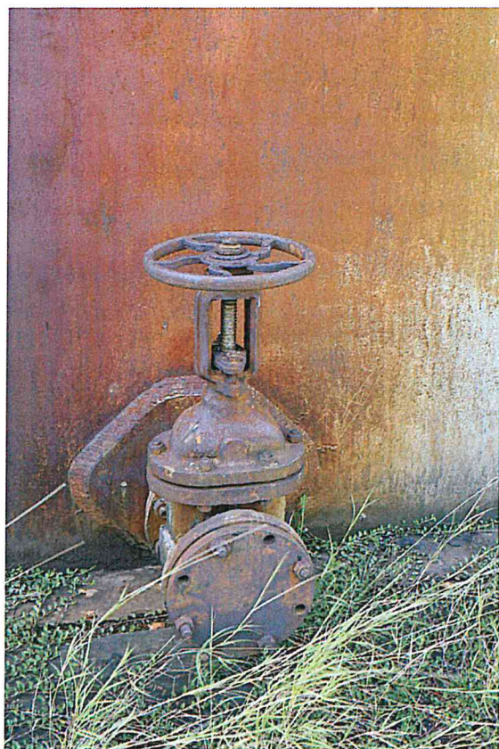
Figure B-27. Valve at ground level of Tank 129, with 4 of 8 bolts missing from blind flange.
