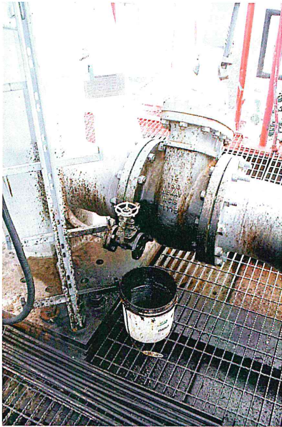
Figure B-17. Drain valve used at Loading Arm, due to MLA No. 3 Vent Valve failure.
