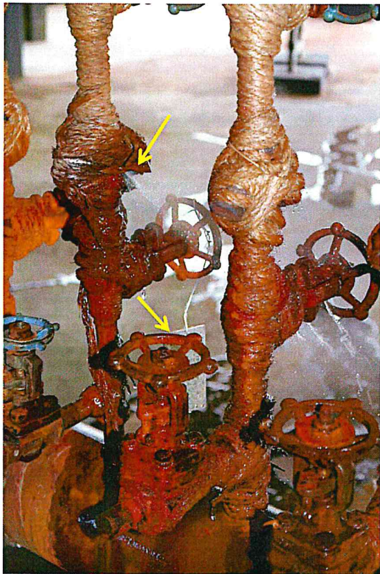
Figure B-48. Fluid (presumably water) leaking from manifold near Visbreaker Heater in 2VBU. Note the aluminum tag related to the "steam tagging initiative".
