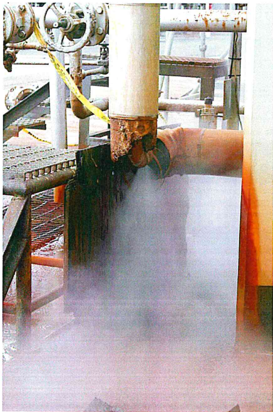
Figure B-72. Steam leak from insulated pipe under Depropaniser Bott. Cooler 931 (rear side.)
