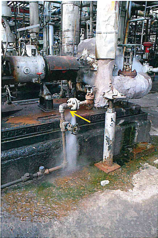
Figure B-61. Example of steam leak at flange at 8CDU.
