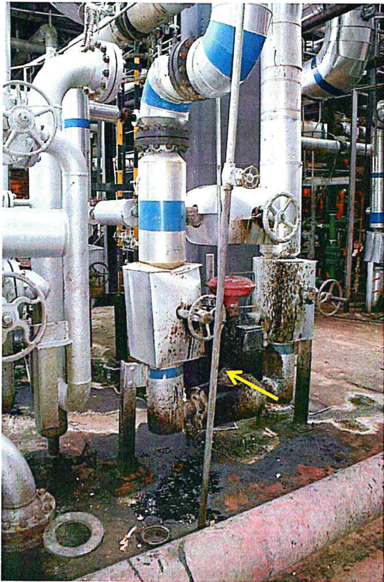
Figure B-44. Unlabeled valve area with crude oil leaks and splashes in 4VDU.
