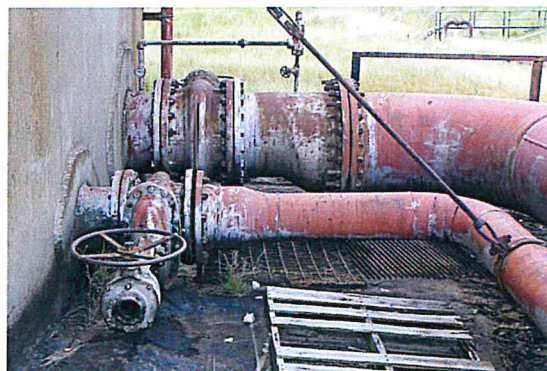
Figure B-29. Example of unlabeled piping and valves connected to Tank 129.
