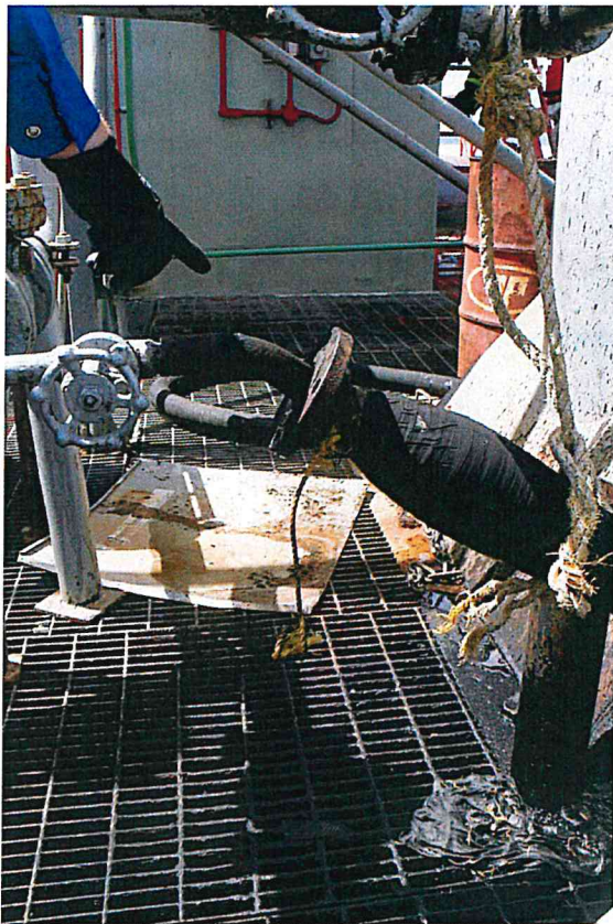
Figure B-20. Temporary hose connection into flanged pipe, with spilled crude to sump.
