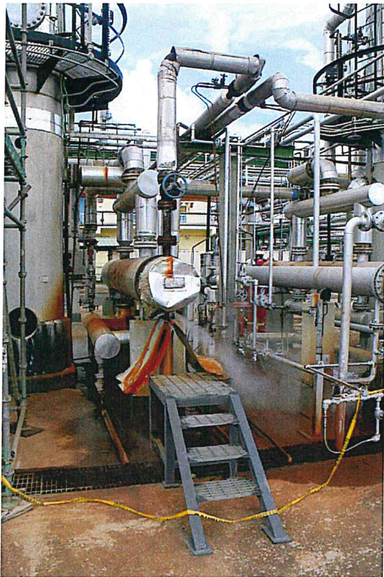
Figure B-75. Steam Leak from insulated pipe of De-Ethaniser Reboiler 930 (rear side.)
