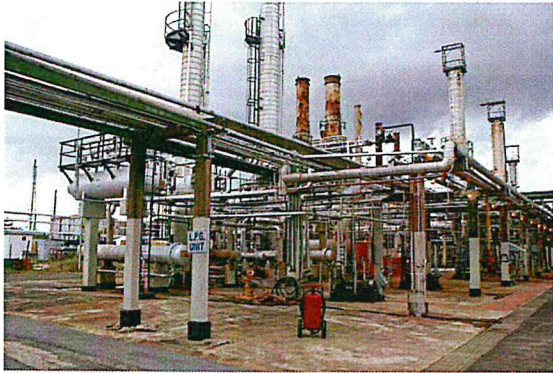
Figure B-64. LPG Unit (front side.)
