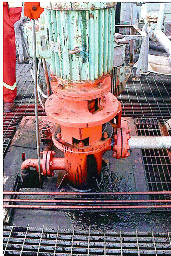
Figure B-18. Sump Unloading Pump, with spilled crude to sump.
