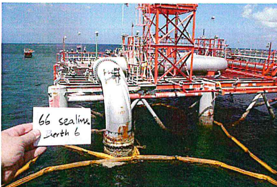
Figure B-12. At Berth 6: Boom in the water around area where Sea Line 66 Clamp was reported.
