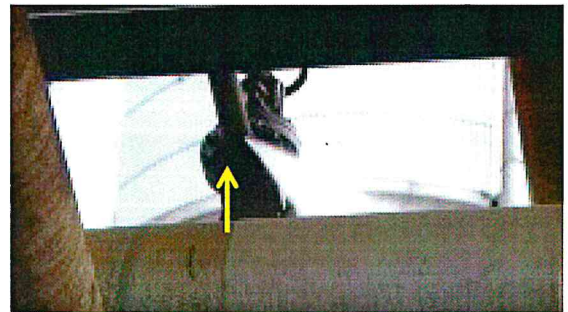
Figure B-51. Close-up of previous photograph, showing steam leak originates at hole in piping.
