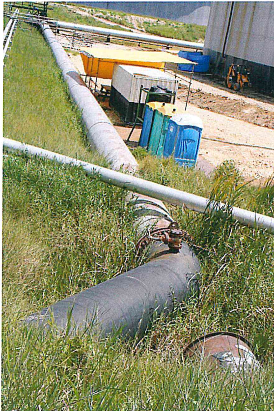
Figure B-34. Line 66 at Bund Area of Tank 100, showing current line (black coating) and previous pipeline 66 (rusty brown.)
