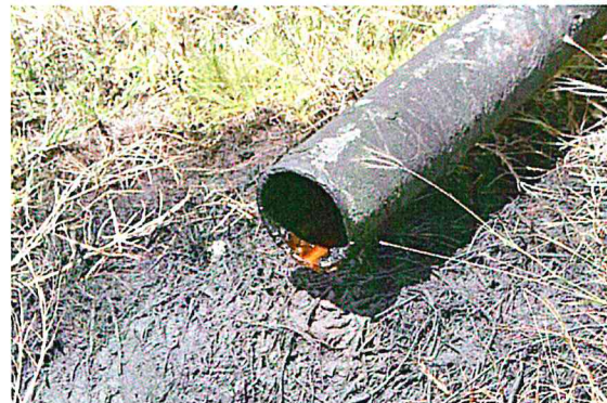
Figure B-26. Close-up of drain line piping from Tank 129, showing wet inside as evidence of ongoing leak.
