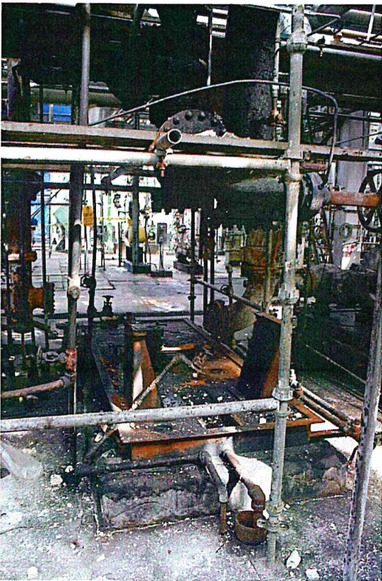
Figure B-58. Foundation of pump that was removed after fire at 8CDU. The surrounding area still shows much fire damage.
