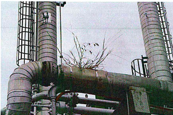
Figure B-66. Plant growing from piping insulation in LPG unit (front side.)
