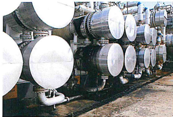
Figure B-55. Equipment C5220A-D at 8CDU.
