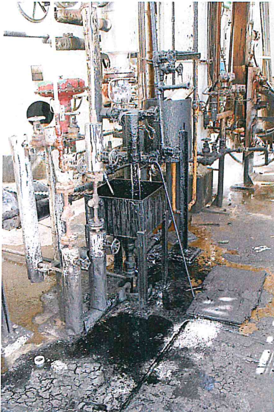
Figure B-46. Unlabeled area with crude oil spill on the ground and covering the equipment.
