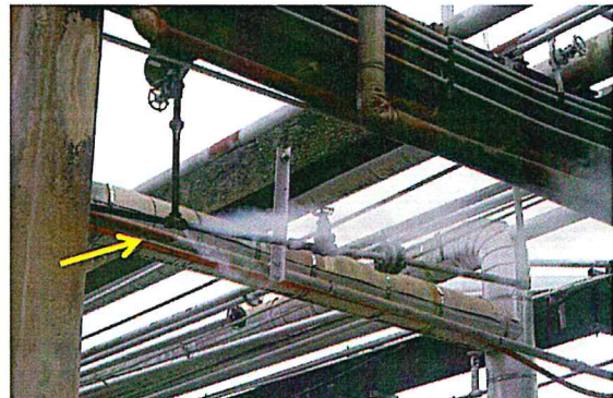
Figure B-68. Example of steam leak at T-fitting in LPG unit.
