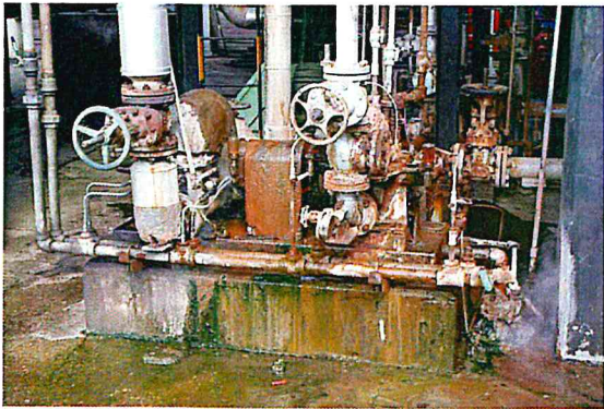
Figure B-57. Unidentified pump at 8CDU with steam leaks and heavy corrosion visible on almost every component.
