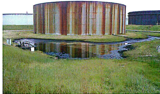
Figure B-24. Tank 129 showing corroded exterior. Bund area around this tank is filled with crude oil and water mixture. The bund of Tank 129 is shared with Tank 103.
