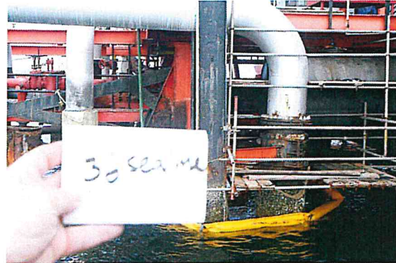
Figure B-8. At Berth 5: Boom in the water and scaffolding above water around area of Sea Line 36 Splash Zone, (no Clamp was reported here.)
