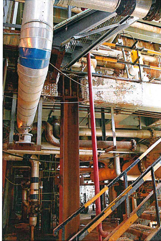
Figure B-38. New structural steel I-beam installed in 4VDU to repair equipment structure.
