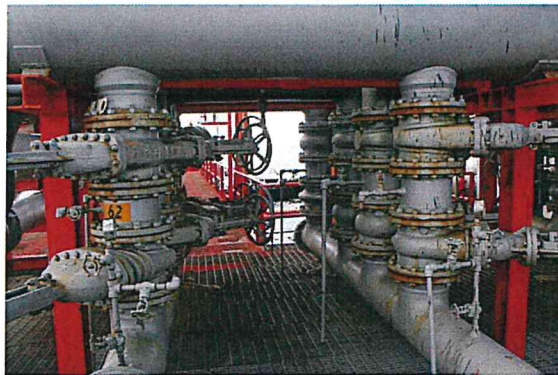
Figure B-21. Pipeline numbers are painted on main manifold at Berth 6, but individual valves are not labeled with unique numbers.
