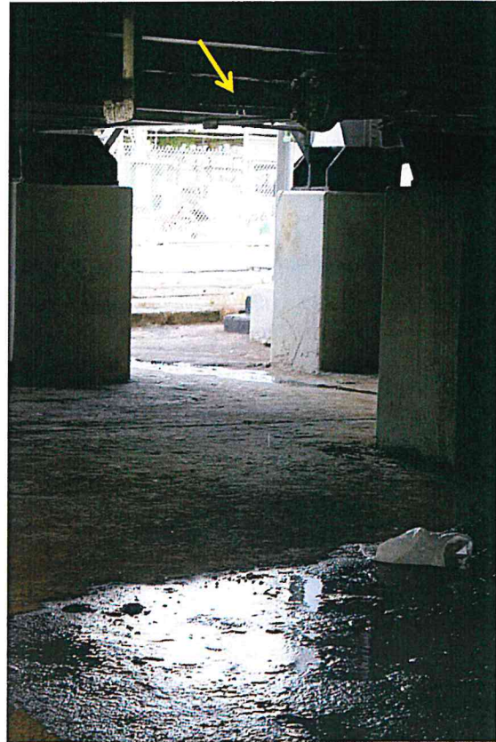
Figure B-43. Continuous leak from piping under furnace in 4VDU (presumably water.)
